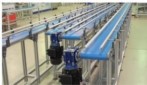
Figure 2.3 Monitoring vibration and temperature in conveyors.
