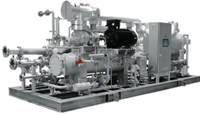
Figure 2.4 Monitoring vibration and temperature in chillers.
